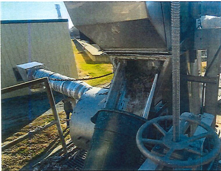
Existing screenings compactor is no longer functioning
