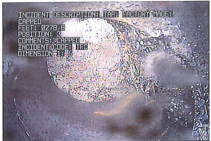
TFC - Tap, Factory Made: Capped @ 278.8 ft. CAPPED
