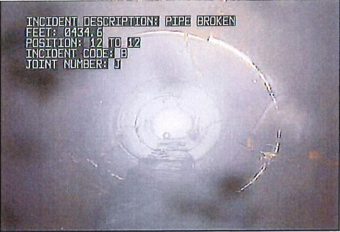
B - Pipe Broken @ 434.6 ft.
