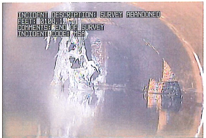
MSA - Survey Abandoned @ 108.1 ft. end of survey
