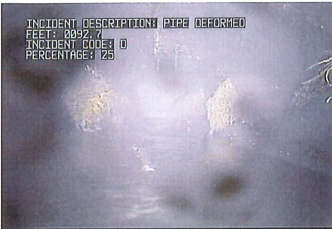
D - Pipe Deformed @ 92.7 ft.
