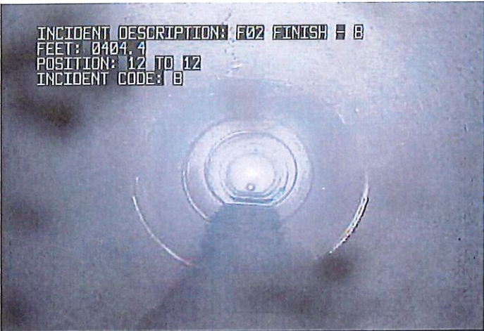
B - Pipe Broken @ 404.4 ft.
