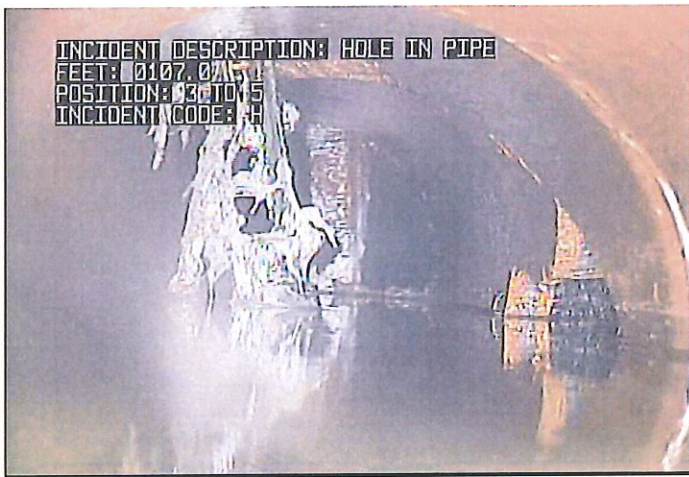
H - Hole in Pipe @ 107.0 ft.
