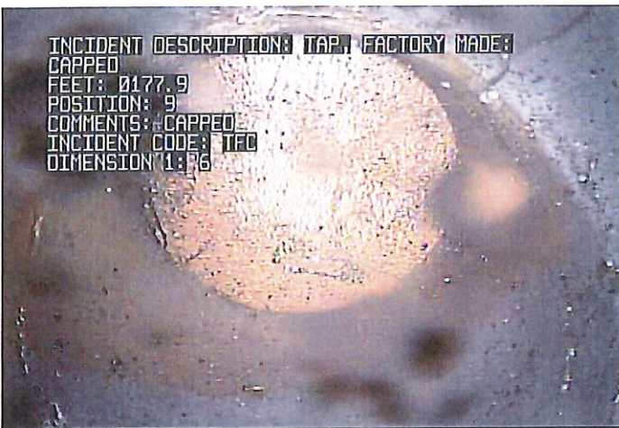
TFC - Tap, Factory Made: Capped @ 177.9 ft. CAPPED
